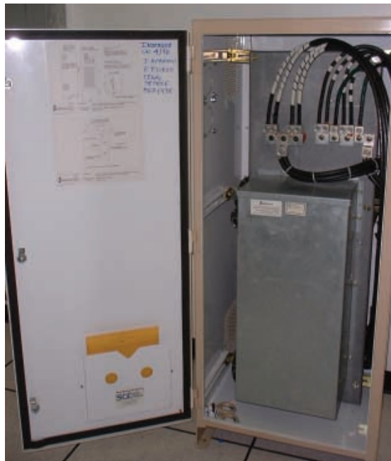
This harmonic suppression system was the answer to one facility's problem.
