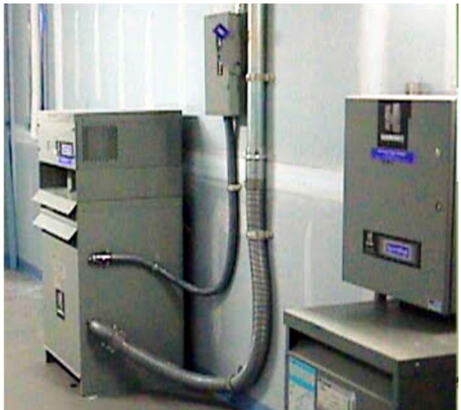
A typical installation August 2004
